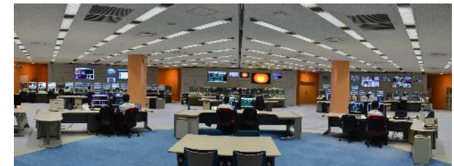
IPC Control Room
